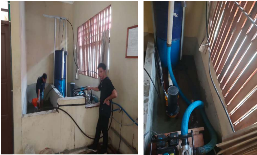
Gambar 3. Instalasi Prototipe Hydram Pump di Laboratorium
