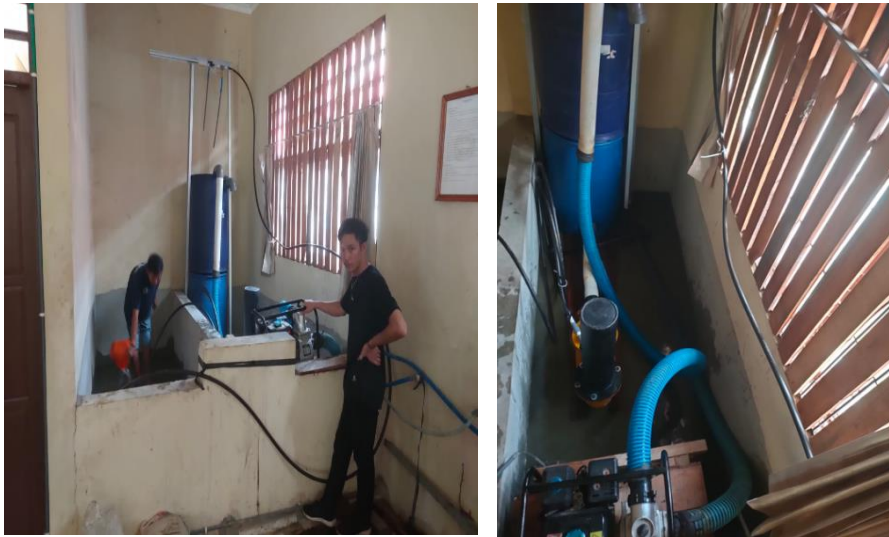
Gambar 3. Instalasi Prototipe Hydram Pump di Laboratorium
