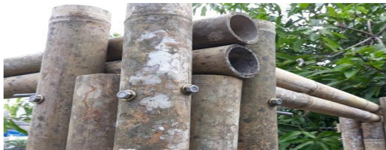
Figure 6. Detailed Images of Ring Balk Construction Applications Simple and Healthy Sustainable Houses Made of Central Kalimantan’s Local Bamboo.
