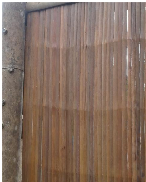
Figure 7. Detailed Images of Construction of Simple and Sustainable Wall Covering Houses Made of Central Kalimantan’s Local Bamboo.
